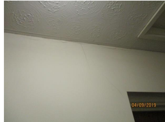
Photograph (18) - Cracking to the hallway, Block 1-6
