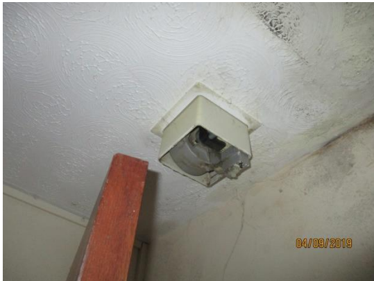
Photograph (15) - Damaged extraction fan, Flat 1
