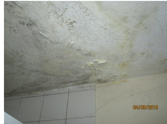
Photograph (12) - Heavy mould causing damage to the Artex ceiling in Flat 1
