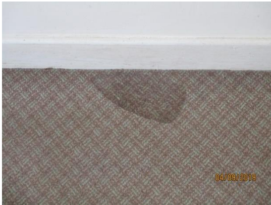
Photograph (11) - Damaged carpet to Flat 1
