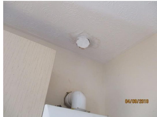
Photograph (16) - Damage to the kitchen ceiling in Flat 6
