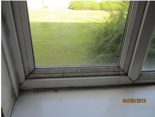
Photograph (13) -Heavy staining to the uPVC windows
