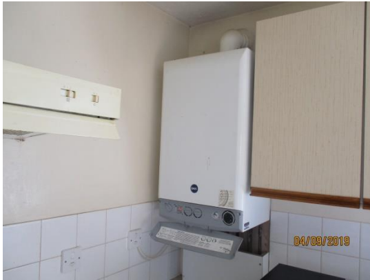
Photograph (9) -General view of the aged gas boiler to Flat 1
