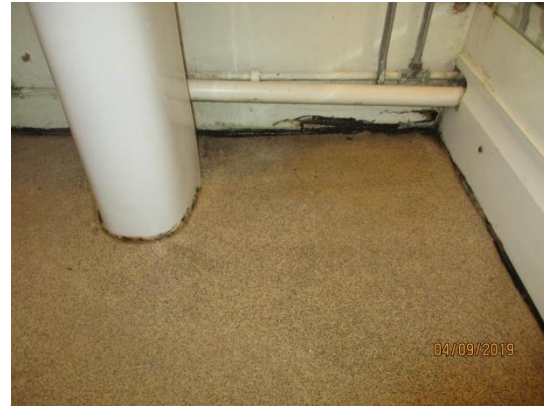
Photograph (14) -Standing water and damage to the bathroom of Flat 2
