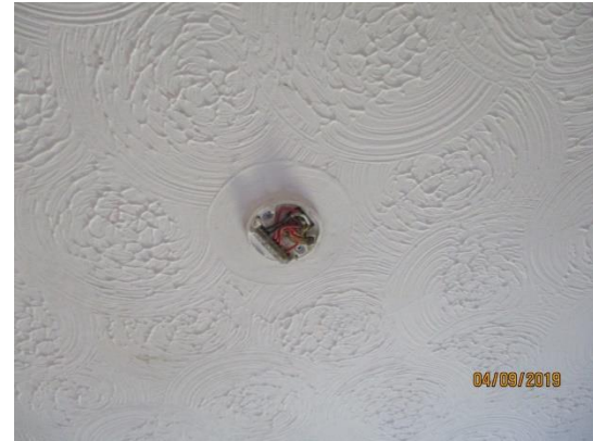
Photograph (10) – Damaged light fitting to Flat 1
