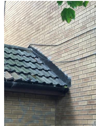
Photograph (24) - Missing flashing to bike store
