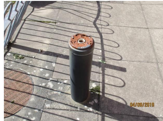
Photograph (20) - Damaged light fitting to external area
