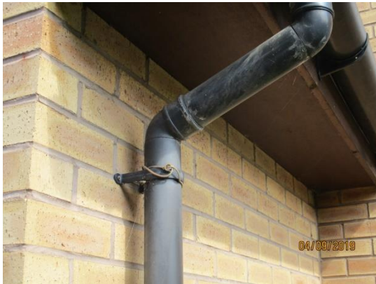
Photograph (19) - Leaking to uPVC downpipes
